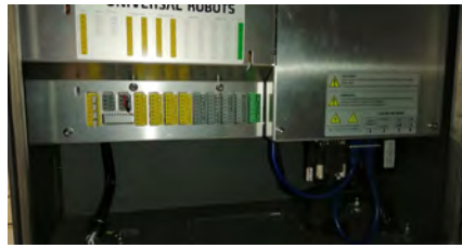
(b) Inside the controller we learn about connectors and cables, which are exposed. The left side includes I/O and safety, whereas the right one leads to the main computer.
