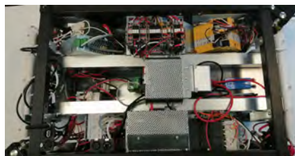
(b) A circuit-breaker switch is present to disconnect the main power line going from the batteries to the rest of the robot. A quick-release connector is also present.
