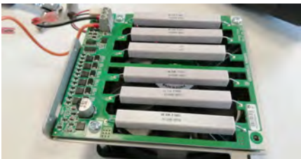
(g) The energy-eater board. This component tends to overheat a fair bit and should generally be checked in case of failure for signs of degradation.
