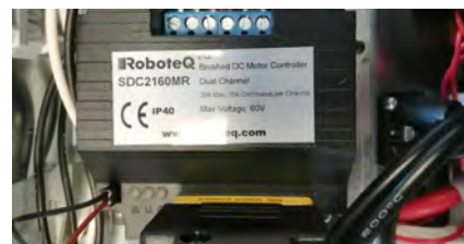
(f) Under the sloped RF cage we find the Roboteq SDC2160, a dual-channel controller for brushed motors with no safe torque (safety) capabilities.
