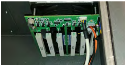
(d) The energy-eater board. This component tends to overheat a fair bit and should generally be checked in case of failure for signs of degradation.
